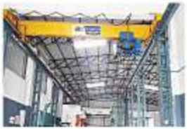
Single Girder Crane (10 Ton)
