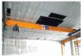
Single Girder Crane (5 Ton)
